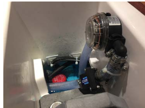
Picture showing filter and non-return valve electrical sump pump.
